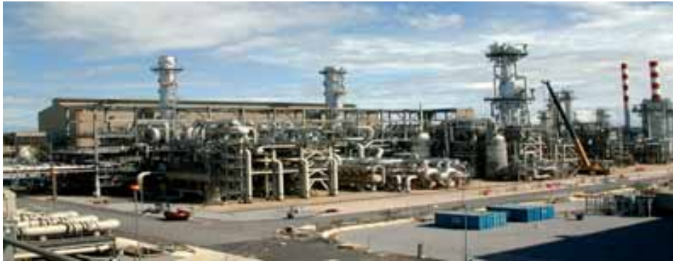
Figure 1.4. The first LNG train in operation; seen from the shoreline of Bonny River. Dimensions: 300x140x30 m (LxWxH).
